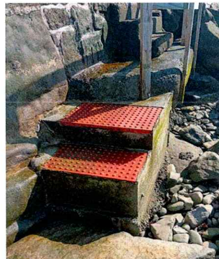
Unauthorized concrete steps with rubber surface
