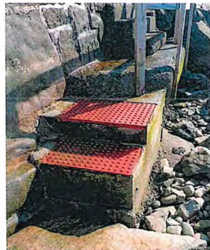
Unauthorized concrete steps with rubber surface
